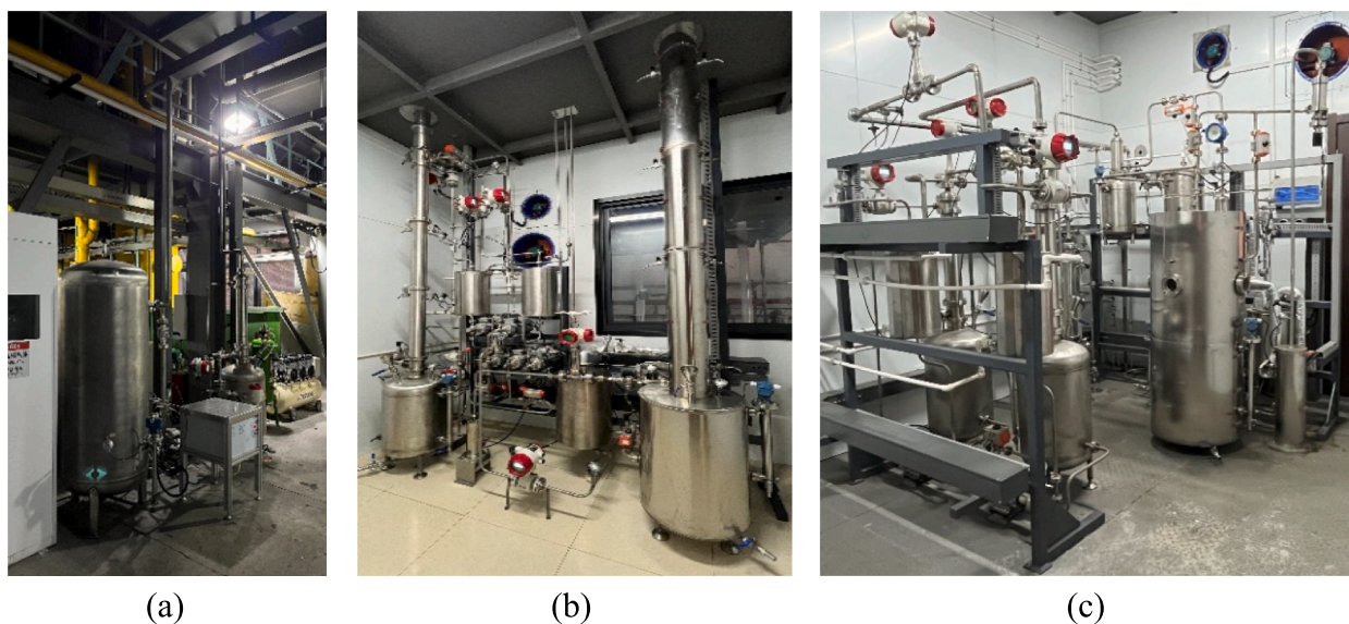
Fig. 2. CO 2 capture pilot plant: (a) first floor (preprocessing unit); (b) second floor (absorption and desorption unit); and (c) third floor (water washing and flash evaporation unit).
